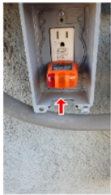
4.2 Item 1 (Picture) main panel
